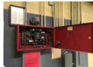
Fire Alarm Control Panel
