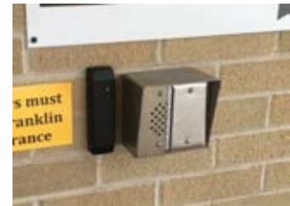
Card Reader & Intercom Box
