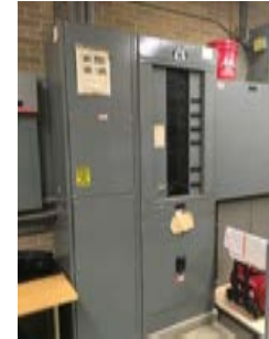
Main Electric Service
