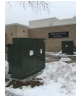
Utility Transformer & C/T Cabinet
